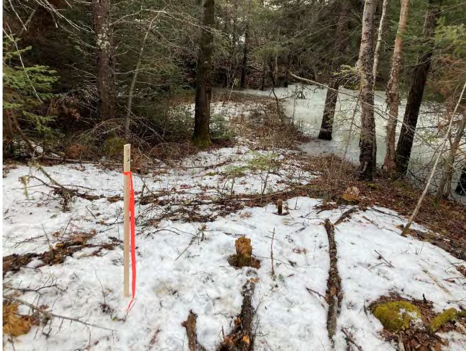
Photo 3: Borehole HF1-04 prior to drilling at Sta. 10+270 (20 m south of proposed CL) looking west, photo taken March 4, 2024
