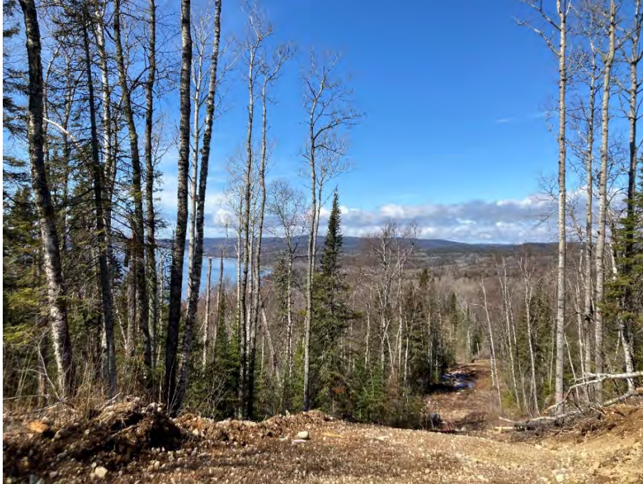
Photo 9: Section DC1 looking west along CL from approx. Sta 12+425, photo taken April 10, 2024
