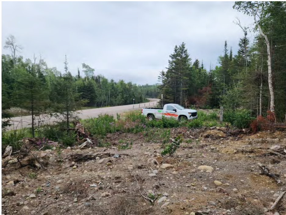
Photo 10: Section DC1 looking east along CL from approx. Sta 12+475 towards Highway 17, photo taken August 16, 2023
