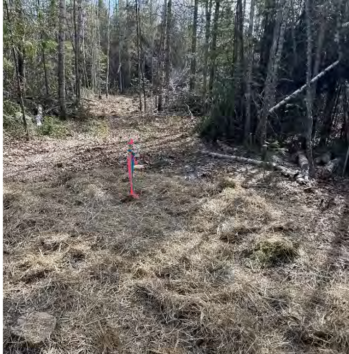
Photo 1: Borehole HF1-01 after completion of drilling near Sta 10+275 looking south, photo taken March 18, 2024
