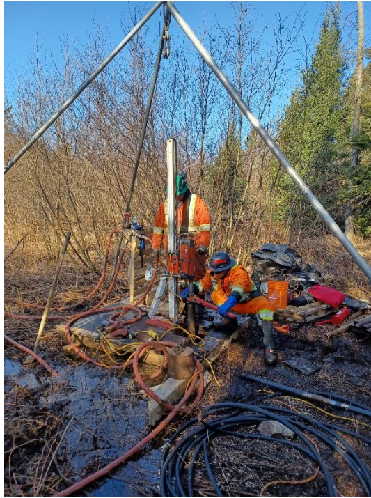
Photograph 3. SPT sampling at SW2 at borehole BH2-6 using tripod setup in swamp (April 09, 2024)
