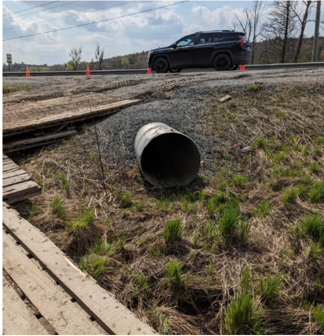
Photograph 11. Corrugated steel pipe culvert inlet and east side of embankment, facing west (May 7, 2024)
