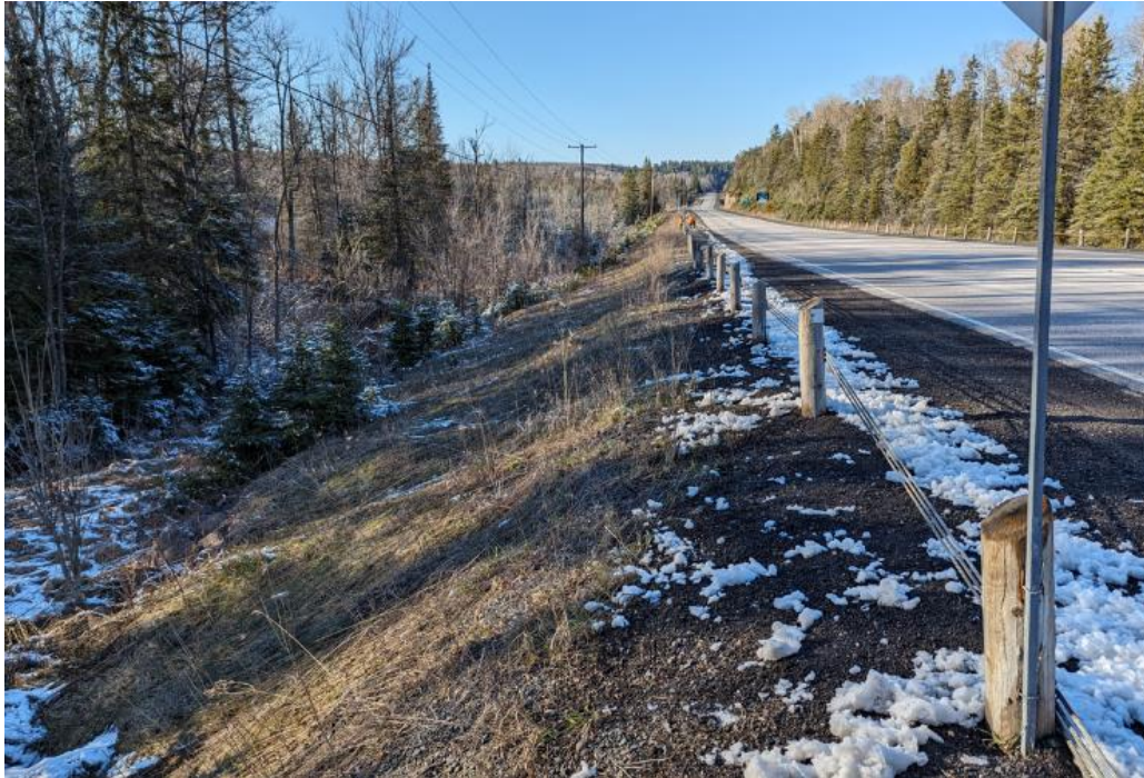
Photograph 1. Roadway surface and shoulder, embankment side slope, and ground conditions beyond embankment toe along SBL (west) side, looking north (April 24, 2024)
