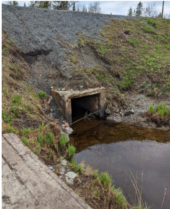
Photograph 8. Concrete box culvert inlet and east side of embankment, facing west (May 7, 2024)
