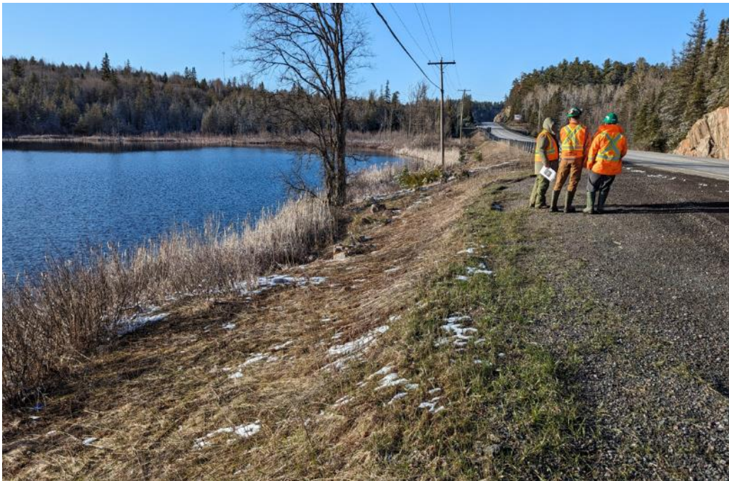
Photograph 2. Roadway surface and shoulder, embankment side slope, and ground conditions beyond embankment toe along SBL (west) side, looking north (April 24, 2024)
