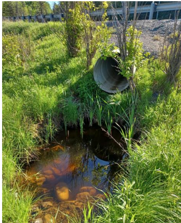
Photograph 12. Corrugated steel pipe culvert outlet and west side of embankment, facing east (May 7, 2024)
