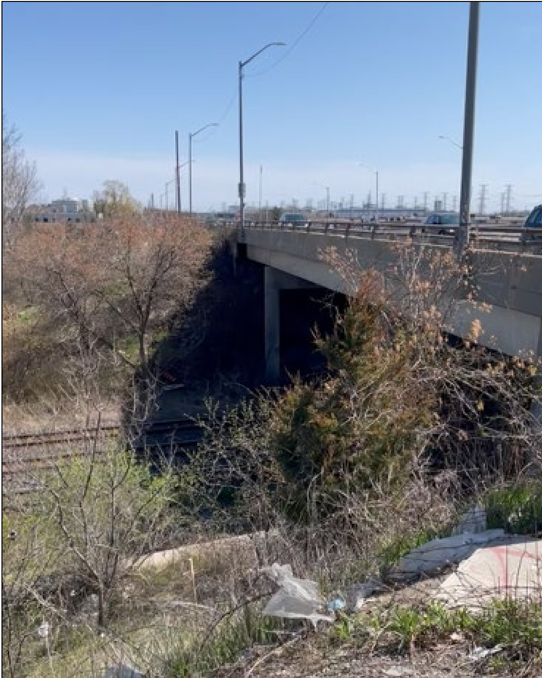
Photo 4- Pier 1 and south abutment of Brock Road and CN Overhead (looking south) Date: May 2022
