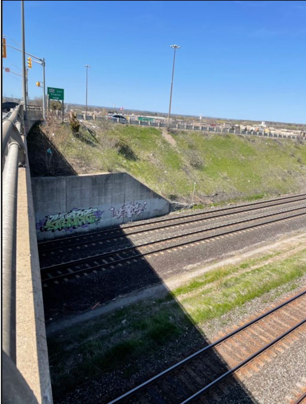
Photo 2- Northeast side of Brock Road and CN Overhead (looking north) Date: May 2022
