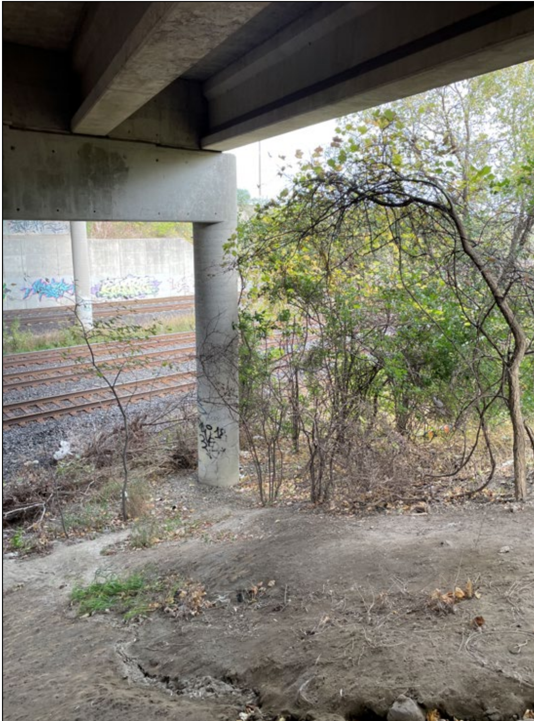
Photo 5- Piers 1 and 2 of Brock Road and CN Overhead (looking north) Date: May 2021
