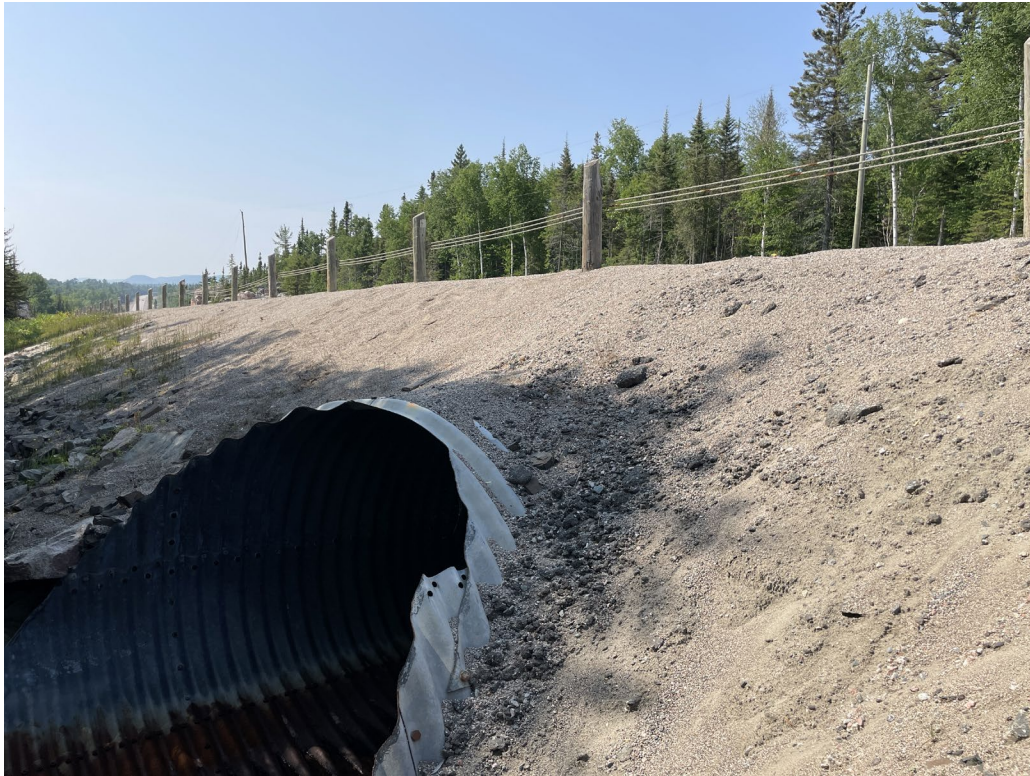
Photograph 1: Highway 17 – Clay River Culvert – Embankment West Slope at Culvert Outlet, Looking North
