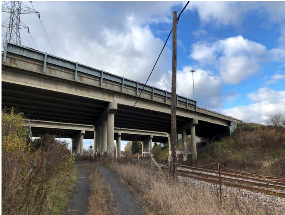
Photograph 3: East of east abutment and piers of Site 3-302/2 (WBL), looking west (November 2018).
